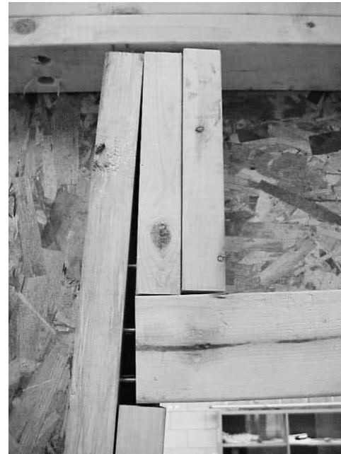
Fig. 12. Example of a separation at one corner of the wall.
